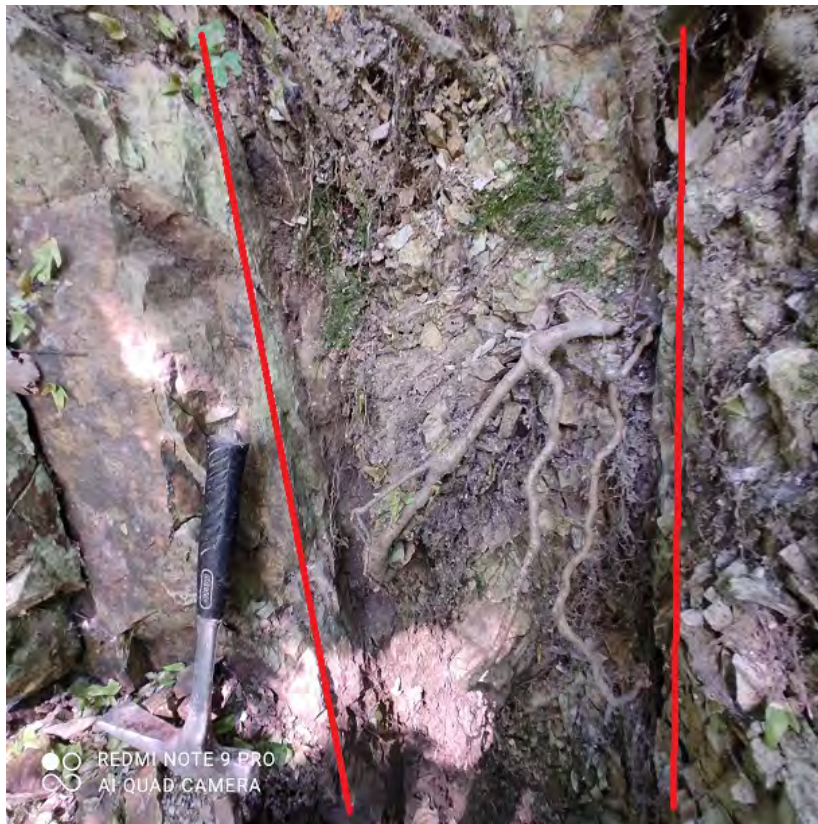
Fig. 3. Fault seam zone (red lines show the L-systems tectonic cracks with slip lines (slickensides))
